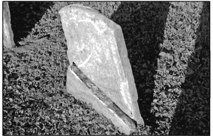
This stone with a simple epoxy repair failed within months of the repair.
