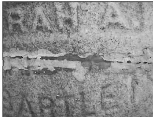
Here the handyman attempted to hide the epoxy repair by using paint to cover the excess epoxy. Of course the effort failed and the stone is even more significantly disfigured.
