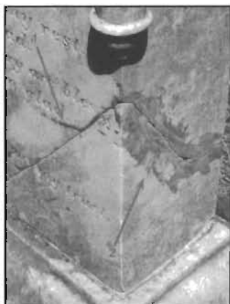
This photo shows a broken obelisk with a “simple,” but very sloppy and unprofessional epoxy repair.
